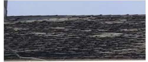
Roof in desperate need of repairs having to be put on hold.
